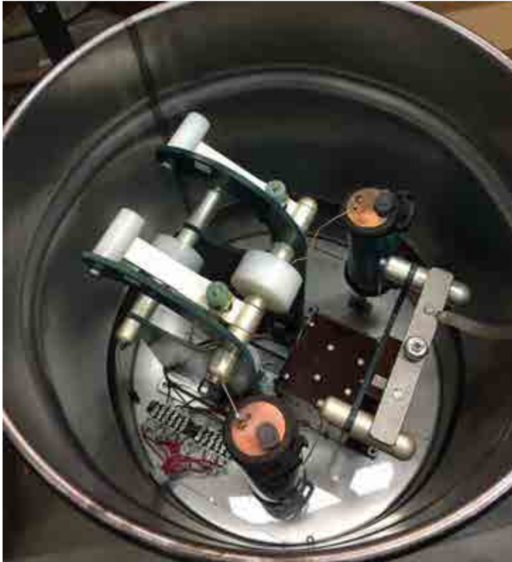
Figure C.5: A 20-gallon oil drum contains the three Ross HV relays used in the charging circuit. The relays are operated by the control panel (see Sec. C.3.1 and Fig. C.4) during the charging sequence. The large copper-sulfate dump resistors in this photograph were ultimately replaced with 50-k \Omega ceramic resistors.
